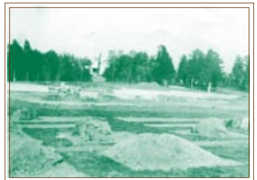
Thomas Sears presented the final drawings for the formal garden to Mrs. Reynolds in the fall of 1917. This photograph shows the East Rose Garden under construction.
